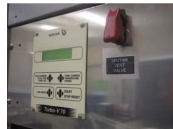
T.P. Controller and Vent Switch (rack mounted)
